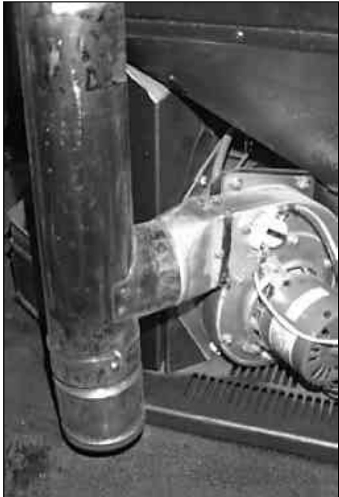
(Figure 11) Clean-Out Cup Connected to Tee
