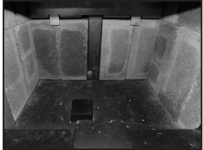
Figure 25: Firebox floor with ash dump.
