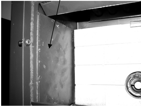
Left side heat exchanger shown
