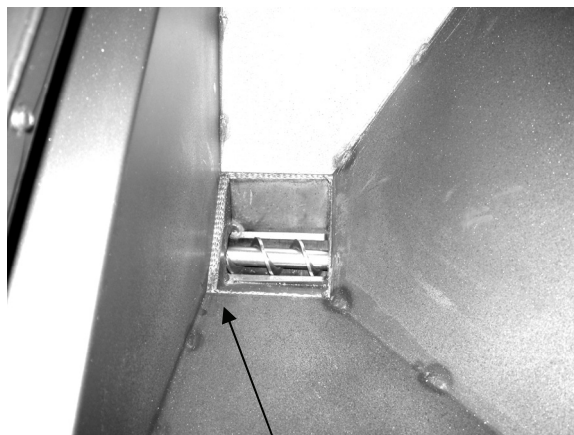
Inside of hopper
