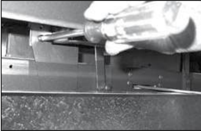
Figure 4.20 Timer Box Installed
