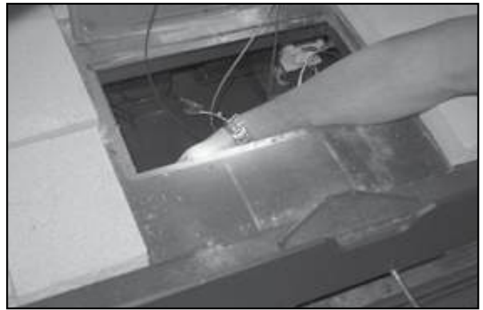
Figure 4.17 Hand in Access Door
