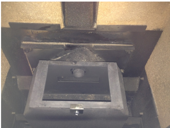
Figure 35: Remove ash from ignitor tube (underneath rept)
