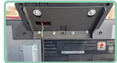
Control Panel Mounting
